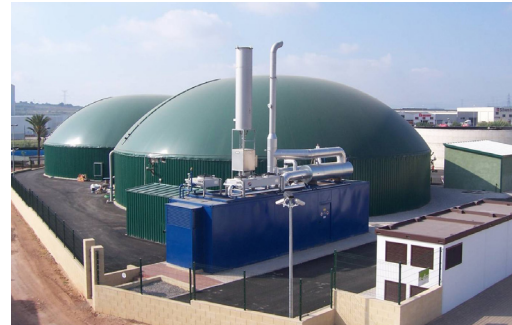
AEMA Bio-gas Plant
